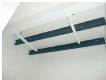
图1 低放射性废水处理设施内的部分房间加固 Fig. 1 Reinforcement of low-level radioactive wastewater treatment facility
